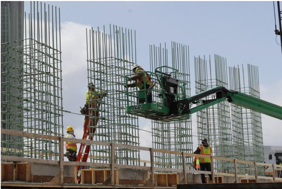
Figure 1 Work continues on a bridge on the Interstate Highway 75 project in Troy, Mich., on April 16, 2020. President Biden unveiled a plan Wednesday to boost spending on major bridges, roads and other infrastructure projects. (Carlos Osorio/ AP)
