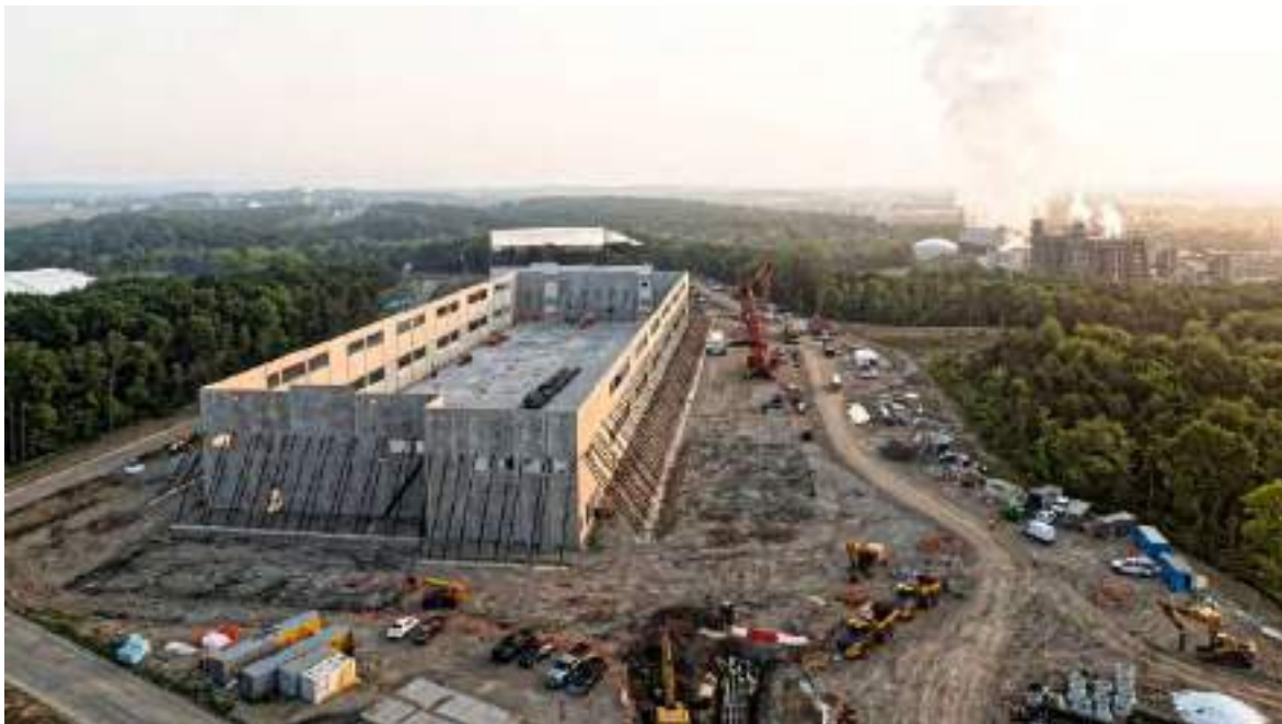
Aerial view of data centers being built in Leesburg, VA. Credit: Gerville/2024
